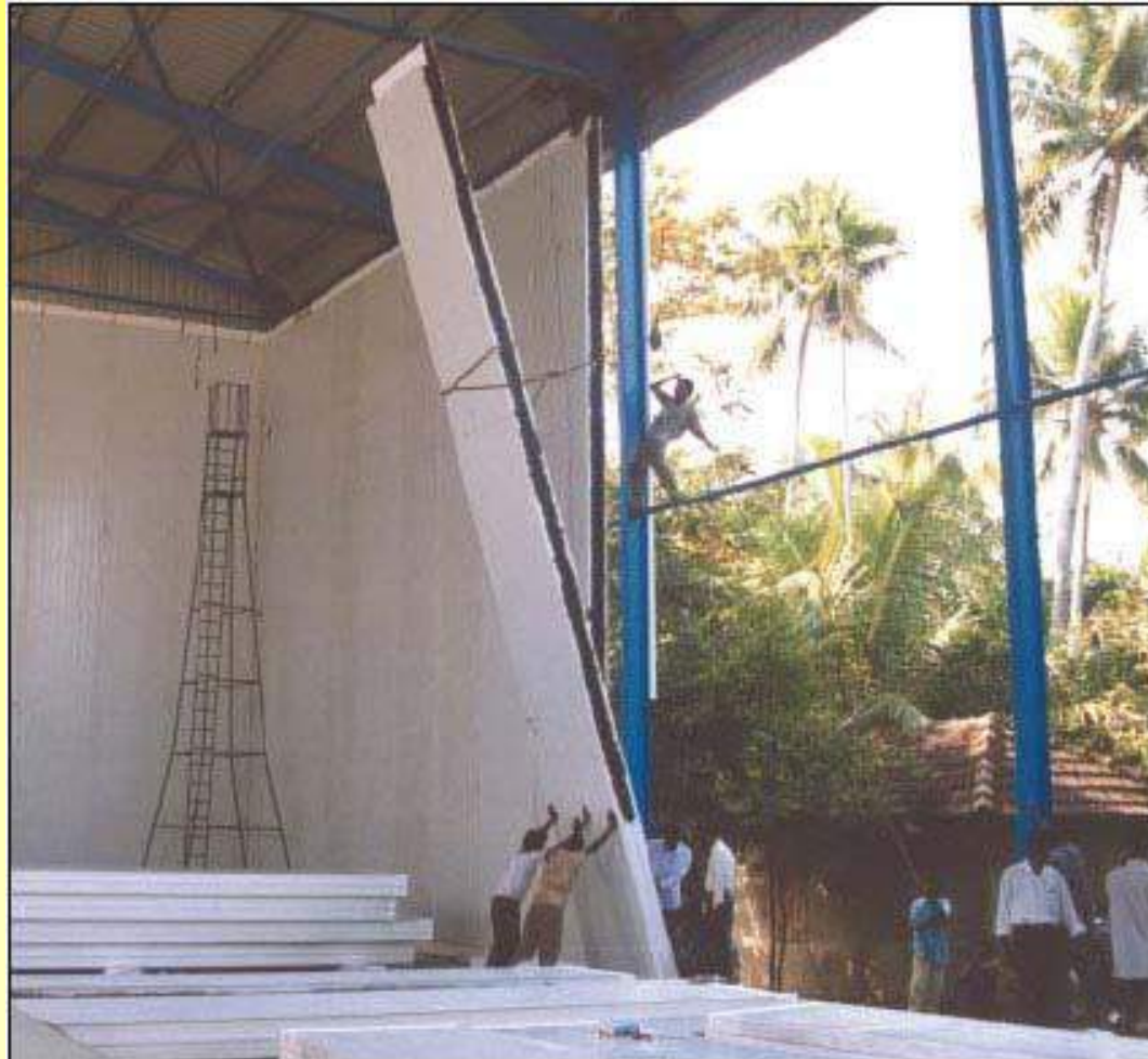
Photo 1 : A large cold store with pre-fab insulated panels under installation for Snowman Frozen Food, Kochi. Room dimensions 50 \times 20 \times 9.5 m high. Photo courtesy of Beardsell Ltd.
